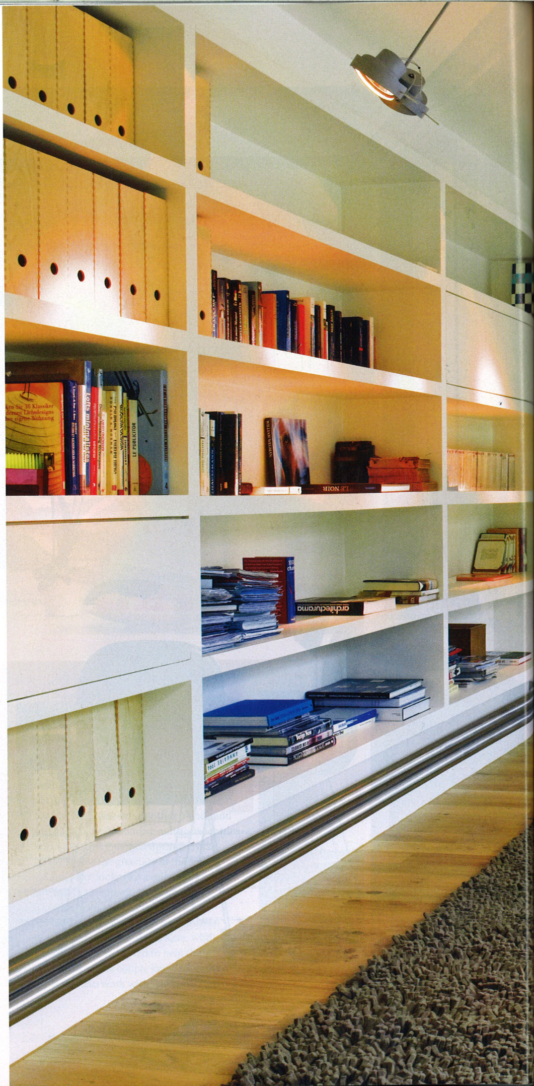
Among the personal rooms on the second floor is a mezzanine space to the double-height lounge below, comprising a library and reading area. The stainless-steel radiator at floor level was specially made for the space and was so long that it had to be tested in a swimming pool. The chair is by Mendini for Cappellini and the bookcases were designed by the architect
